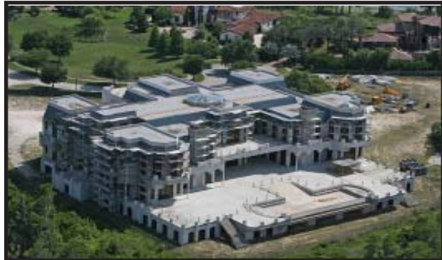
The Versailles house, under construction in 2009, when it was still a mere stump.
